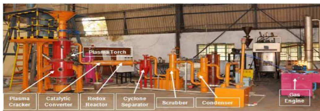
Fig. 2. Plasma gasification plant.
