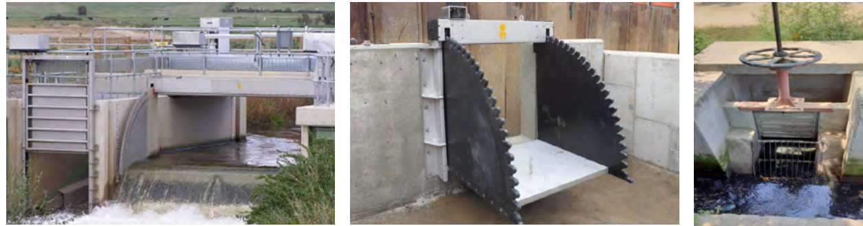
Figure 26: Tilting Weir and Sluice Gates to control flow
