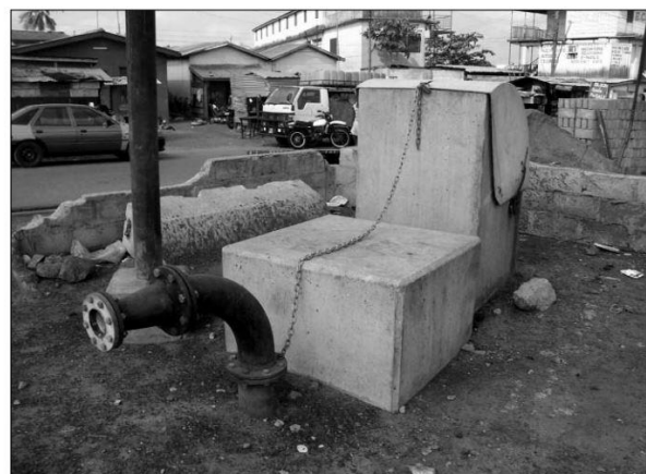
Top of an underground holding tank, showing a chain to lock the lid, a vent pipe and a wall to prevent overflowing excreta travelling onto the road! Source: Boot, 2008
