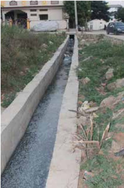
Figure 22: New drains filled with silt and plastics
