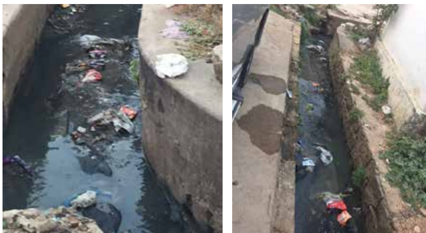
Figure 18: Open Drains in Mehbubnagar
