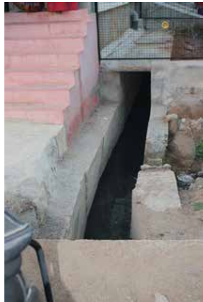
Figure 23: Indiscriminate closure of drains by the households making it difficult to clean
