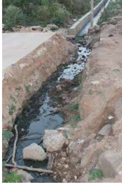
Figure 24: Disconnected drains resulting in stagnation
