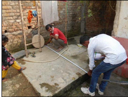
Figure 5: Septic tank in a household
