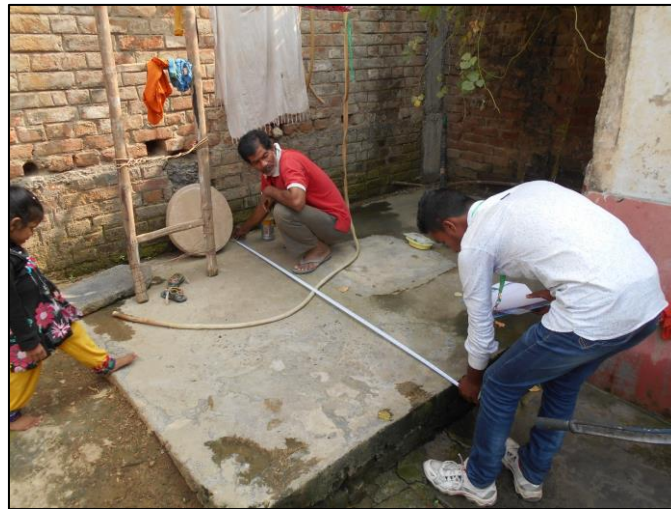
Figure 15: Septic tank in a household
