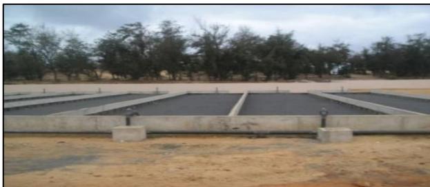
Figure 28: Sludge Drying Bed
