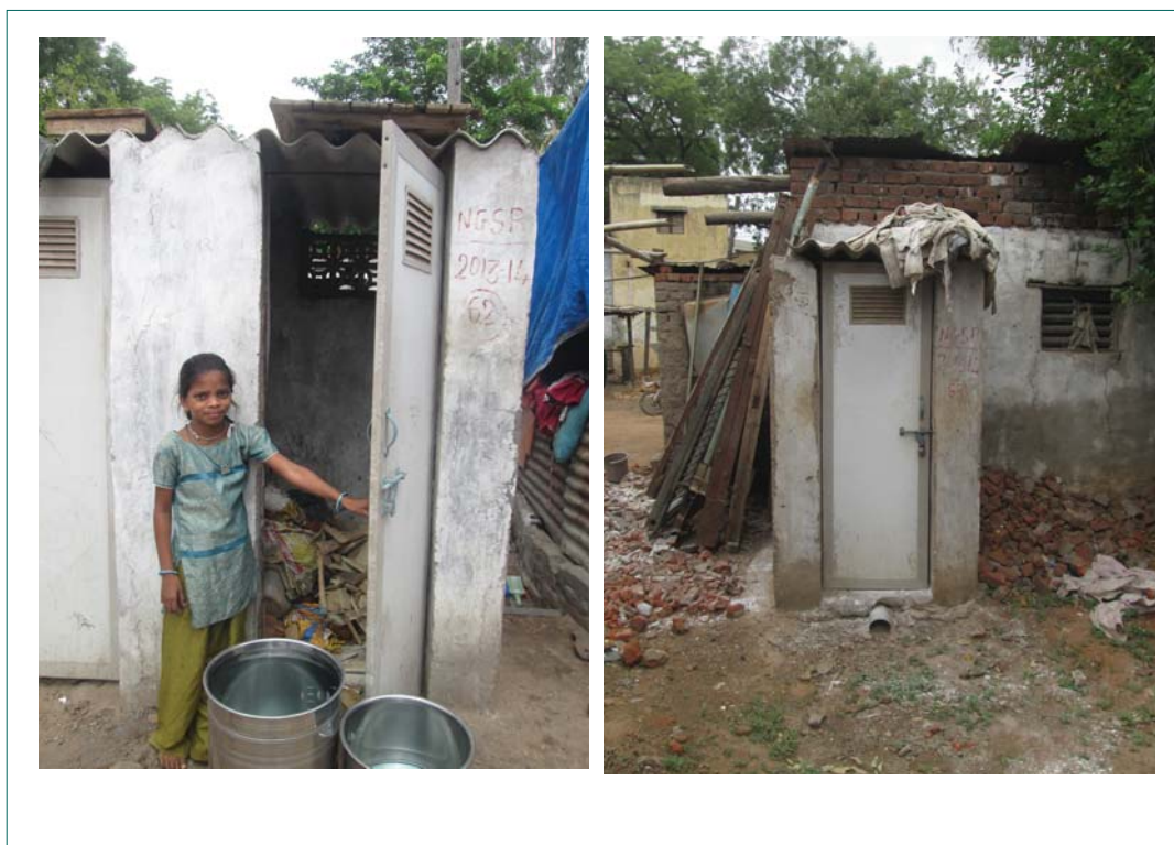
Figure 21: (Below Left) Unused IHHL; (Below Right) Inappropriate outlet for black water at an IHHL
