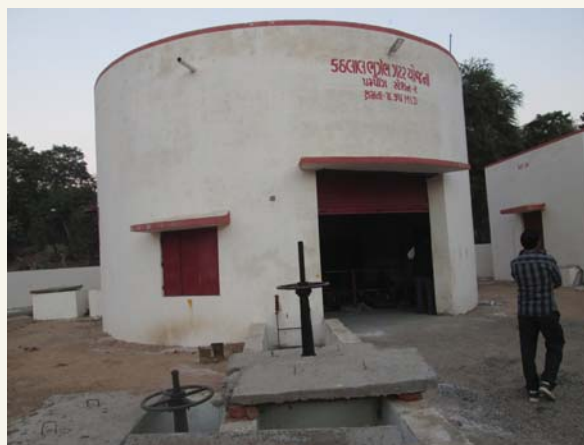
Figure 25: Pumping Station at STP in Kathlal, Gujarat
