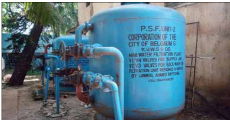
Figure 4: Each open well has been installed with mini water filtration plants which consists of sand filter, alum and chlorine dozer
