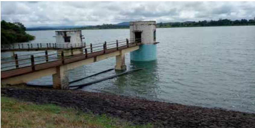
Figure 2: Rakaskop Dam on Markandeya River is a major source of municipal water
