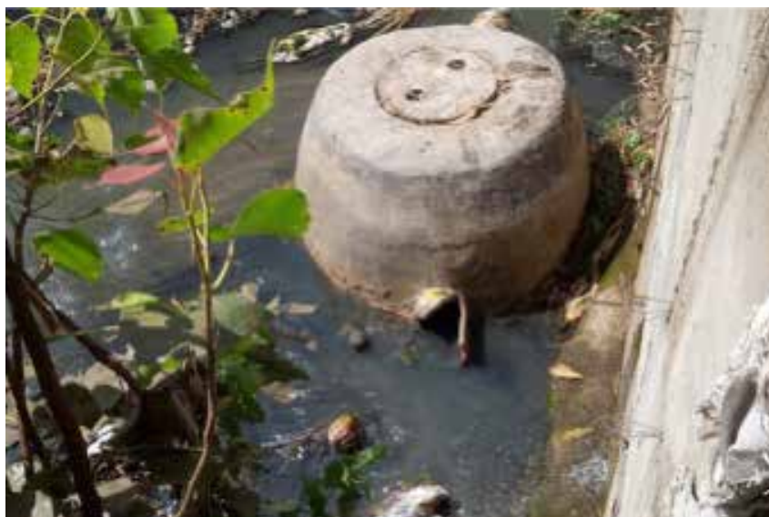
Figure 6: An underground drainage chamber opening into the Belgaum nala
