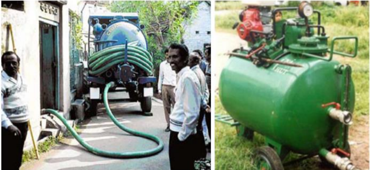
FIGURE 43: VACUUM TRUCK EMPTYING A SEPTIC TANK IN BHARAKPUR NEAR KOLKATA AND A VACU TUG USED FOR EMPTYING SEPTIC TANKS IN CONGESTED AREAS. (SOURCE: EAWAG/SANDEC 2008 & STRAUSS ET AL. 2002)
