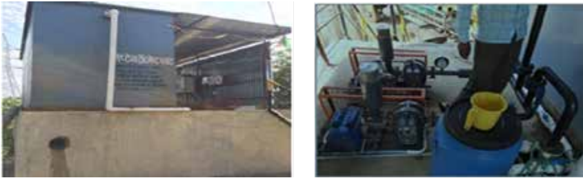
Figure 2.3 Pictures of Jabalpur FSTP
