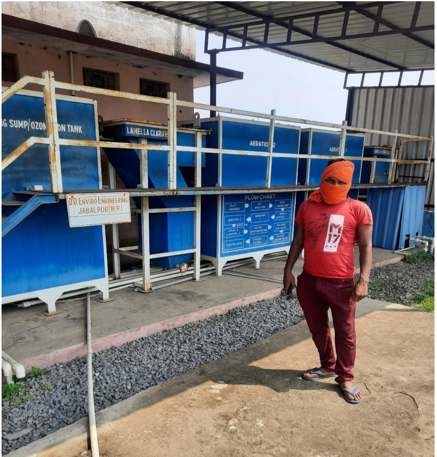
Fig. 9: Faecal Sludge Treatment Plant in Ambikapur
