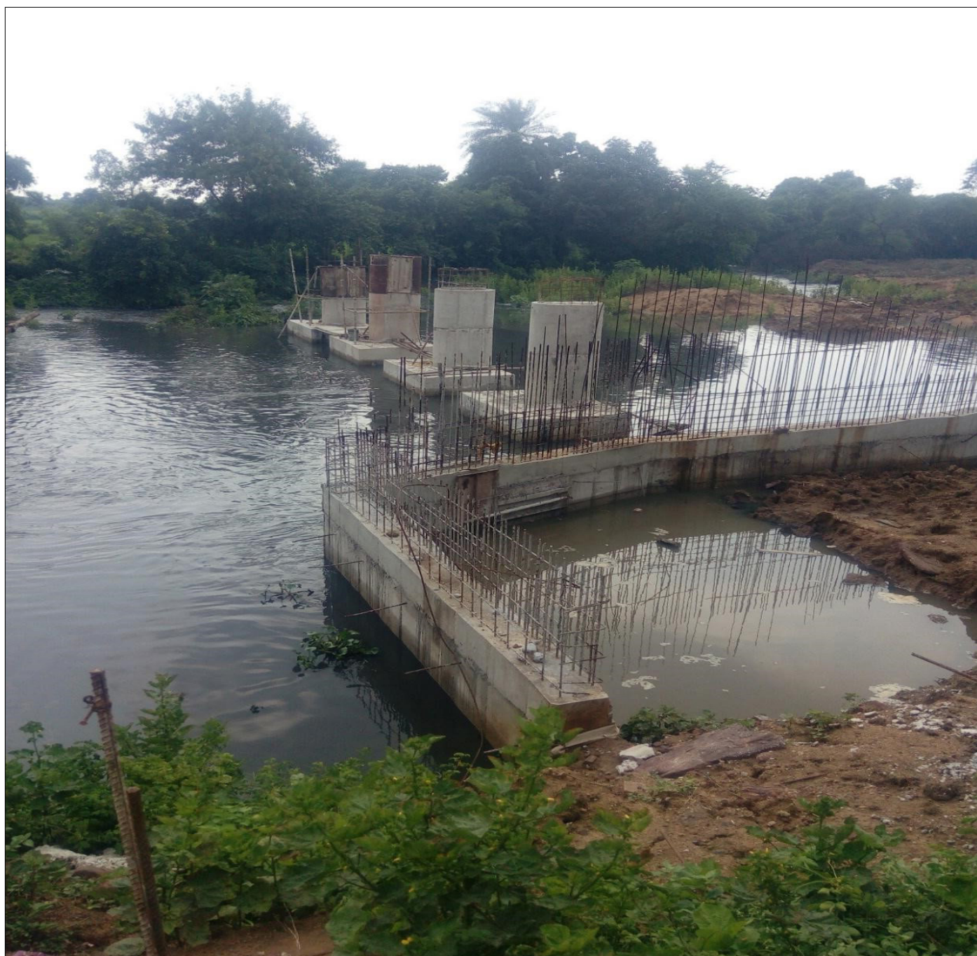
Fig. 15: Structure for diversion of used water from stream to STP at Kara Village
