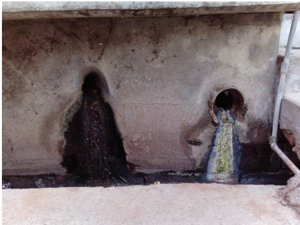
Figure 9: Outlet of a containment unit drains directly into the drains in the street
