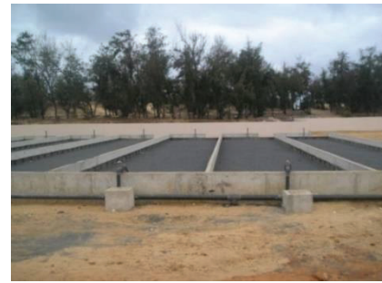
Figure 23 Sludge drying bed
