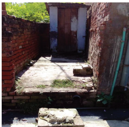
Figure 8: Toilet with Containment Unit
