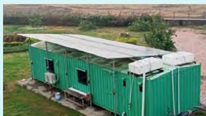
Solar power plant at Sinnar FSTP
