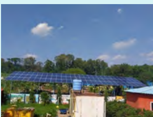
Solar power plant at Wai FSTP
