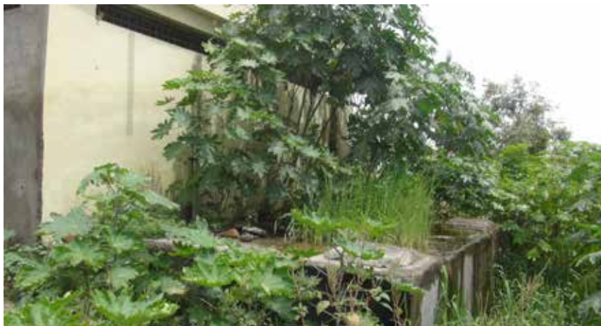
Figure 7: Outflow of Community Toilet in Kacchpura being released into open
