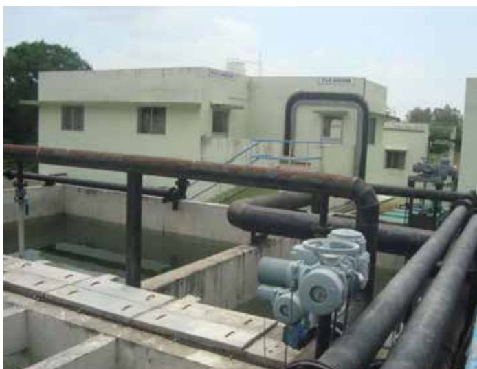
Figure 11 : 12 MLD Sewerage Treatment Plant near Forest Range Office Rewa
