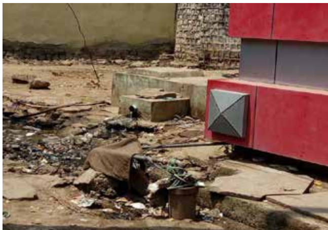
Figure 5. Outflow from Septic Tank of Public Toilet in Bus Stand releasing into the open drain
