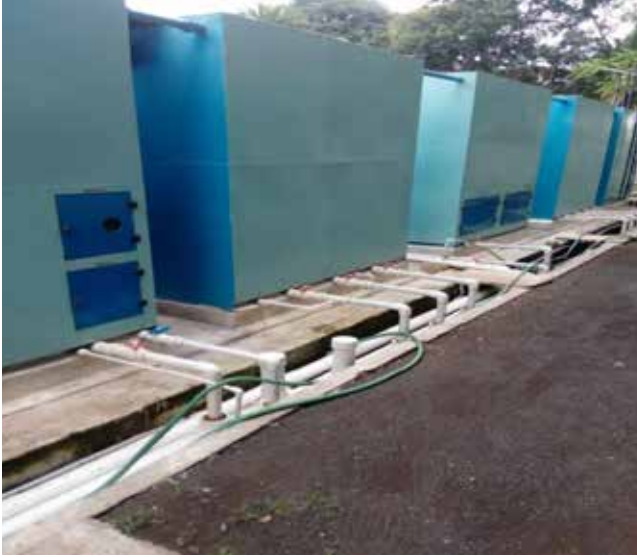
Figure11: The Fluidised Aerobic Bio-reactor STP at Gwari Ghat
