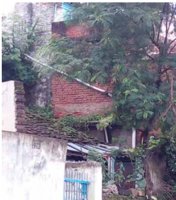
Figure 5: Wastewater pipe from house on top of hill to the open drain below
