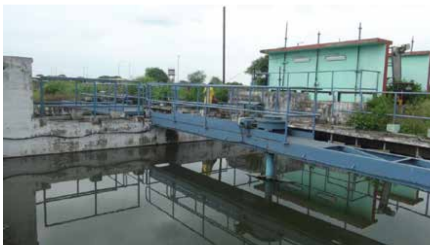
Figure 10: Structure for distributing wastewater to facultative Pond in Kathonda lying idle
