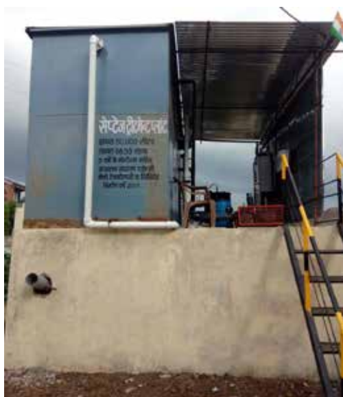
Figure9: Septage Treatment Plant in Awadhपुरi
