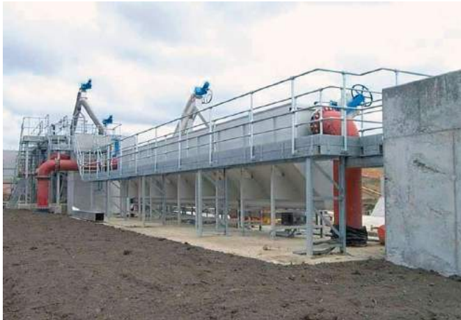
SCBP: Wastewater Treatment Technologies
